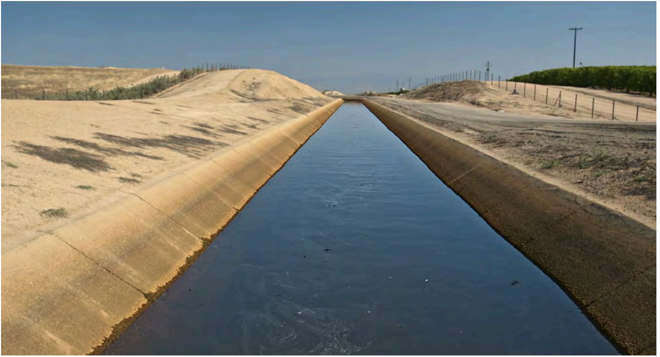
An oil slick on an irrigation canal next to a Wonderful Company orchard
